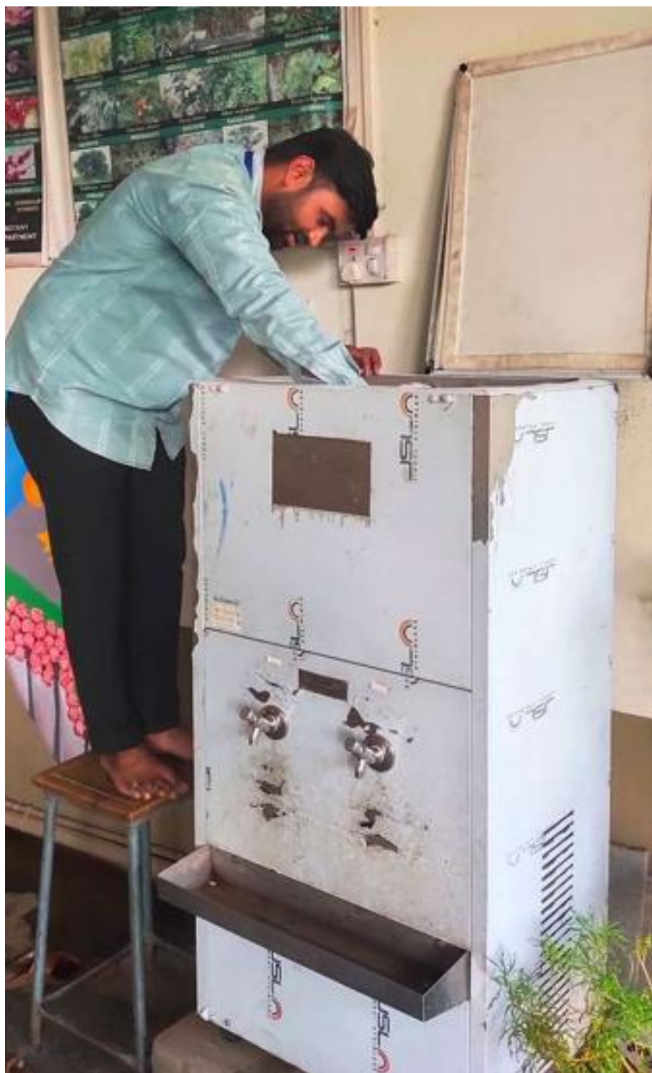
Supporting staff maintaining water cooler
