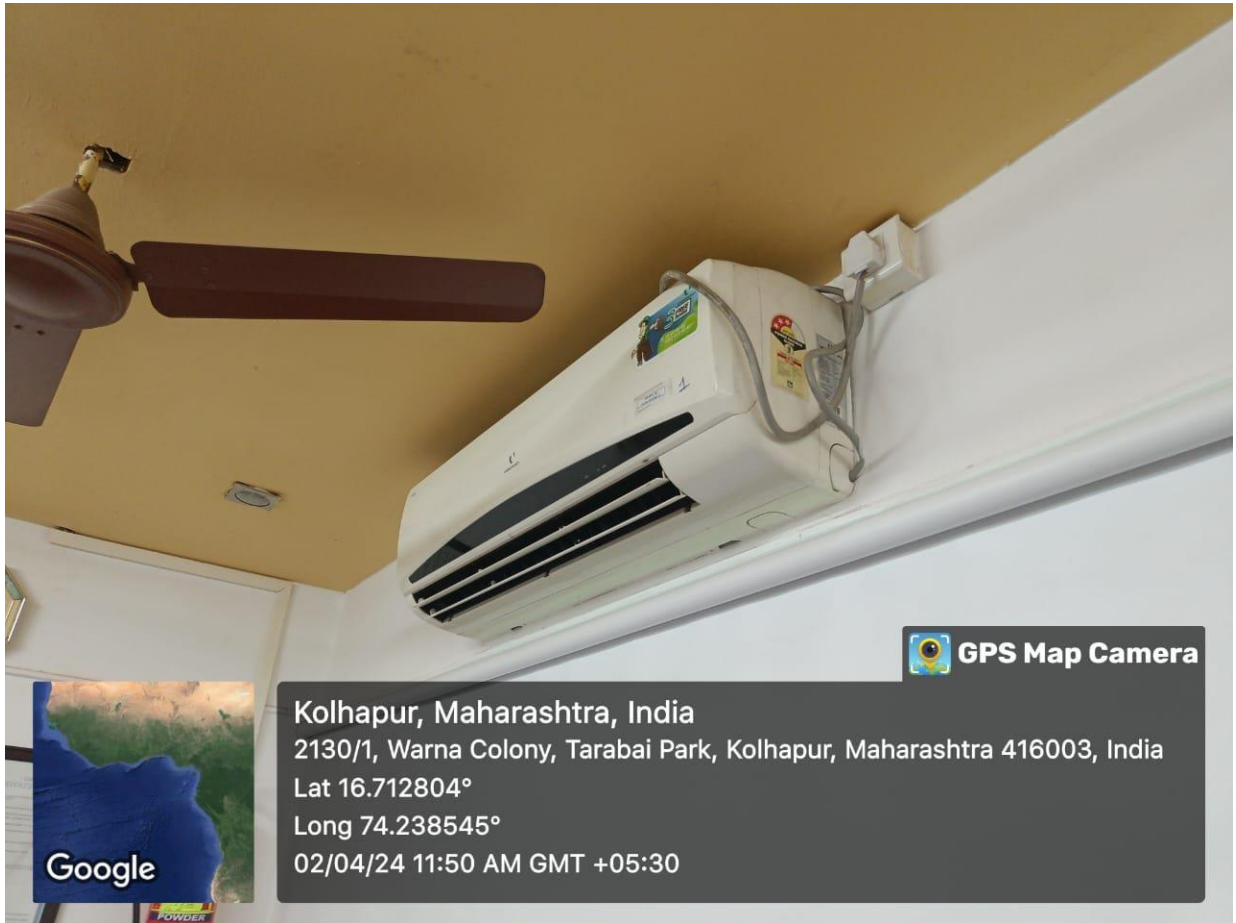
4. 3 star rating air conditioner at computer science department
