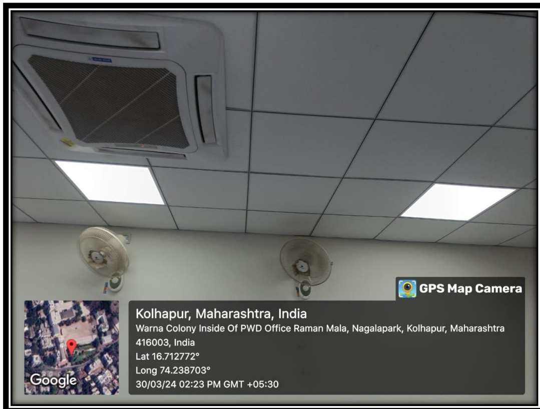
Picture 6: LED bulbs at smart room no.19
