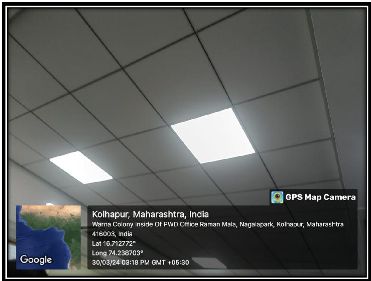
Picture 3: LED bulbs at smart room no.11
