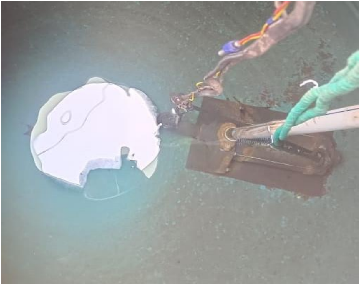
3. Sensor device fitted inside the water tank
