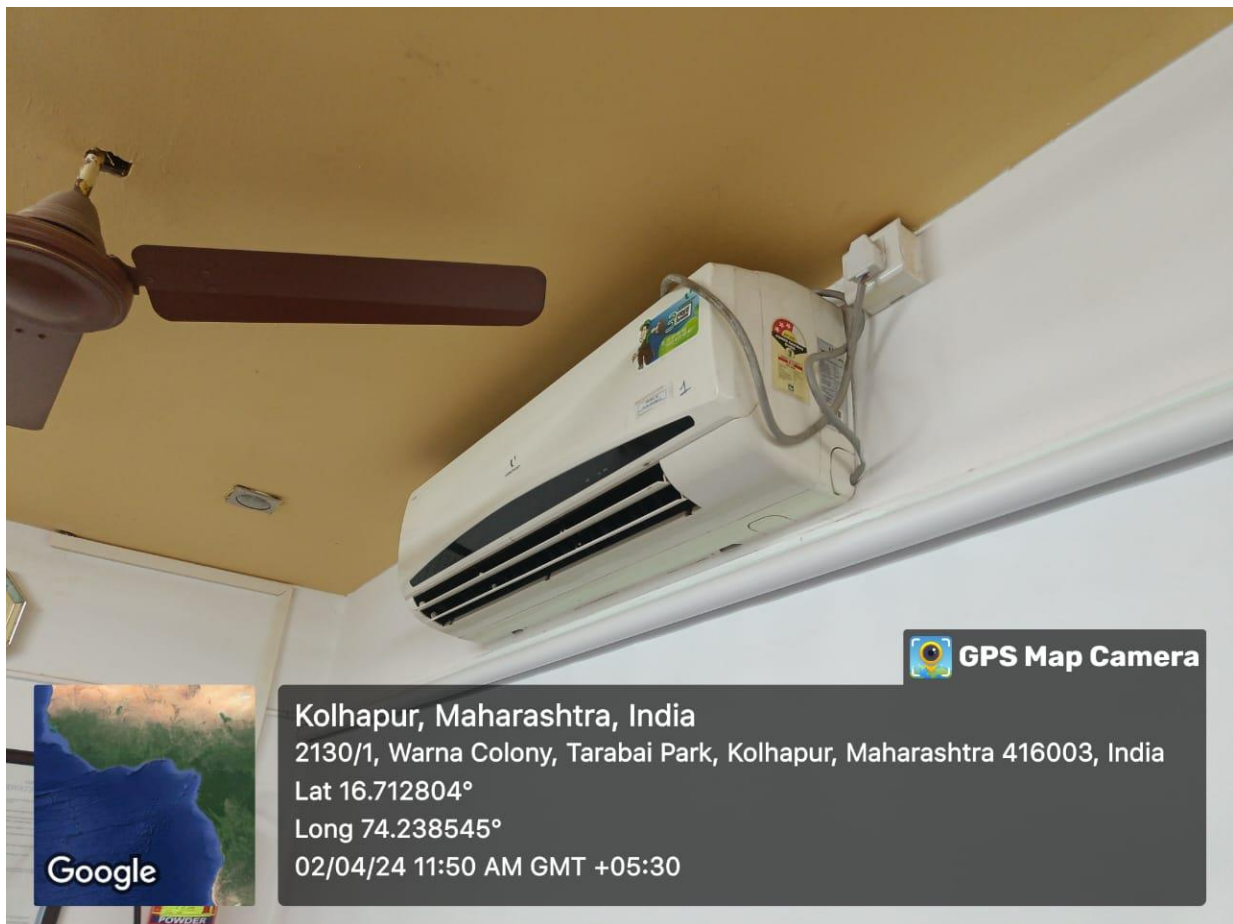
5. 3 star rating air conditioner at computer science department
