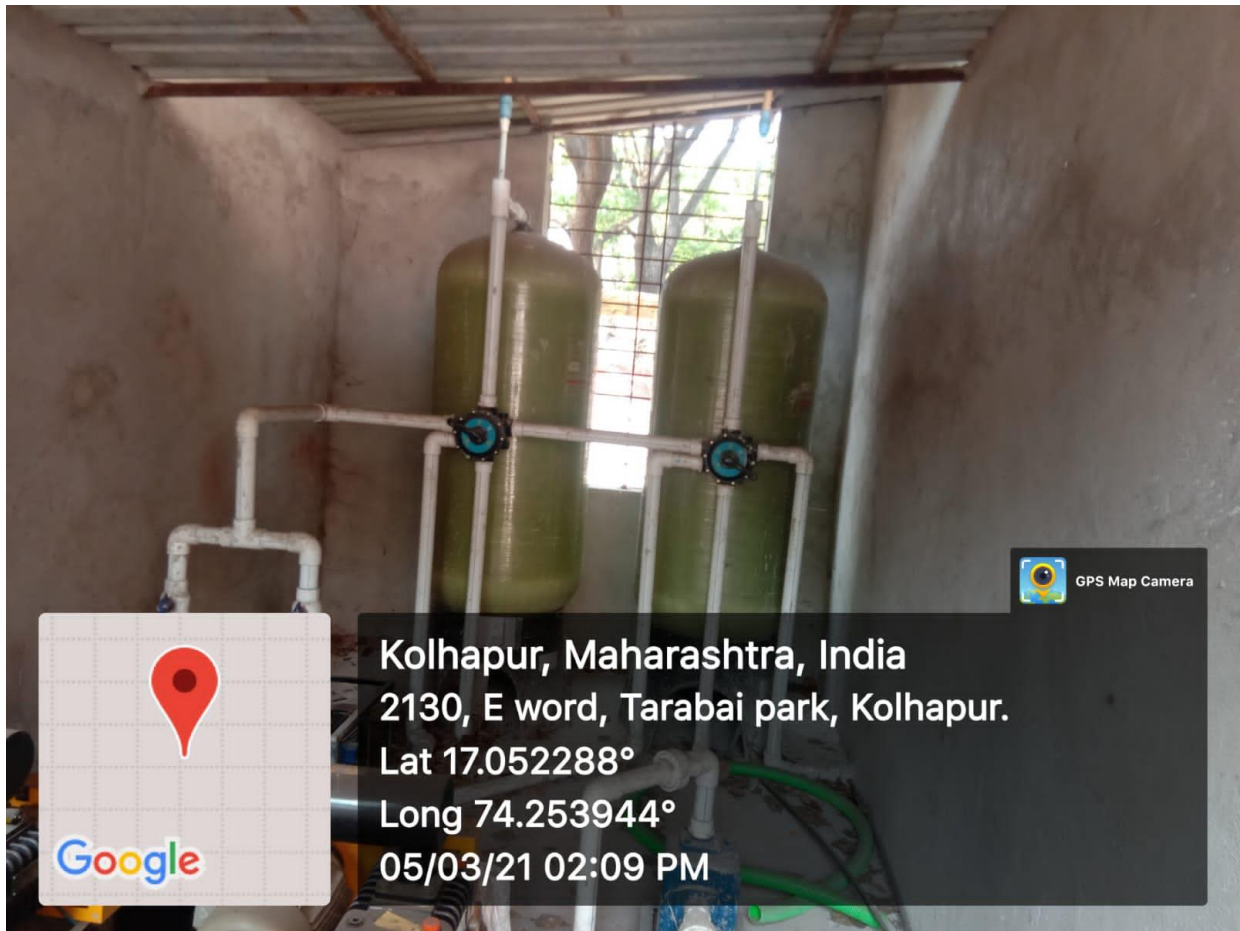
Picture 1. Waste Water Recycling Plant at the Ladies Hostel
