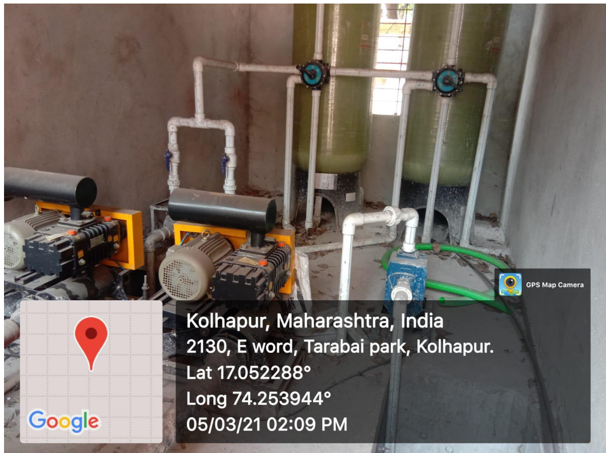
Picture 2. Waste Water Recycling Plant at the Ladies Hostel
