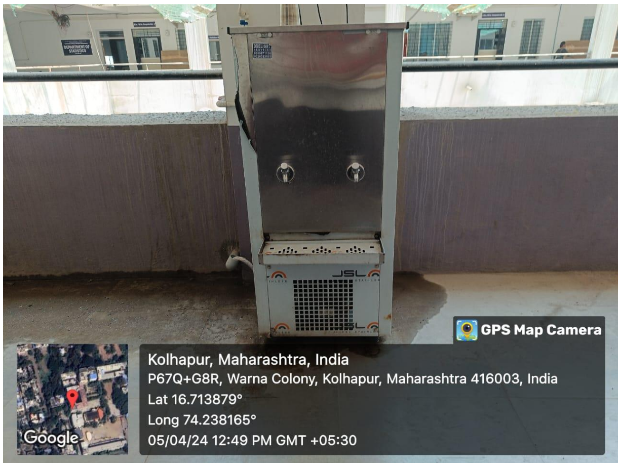
Picture 5. Drinking water facility at Physics department
