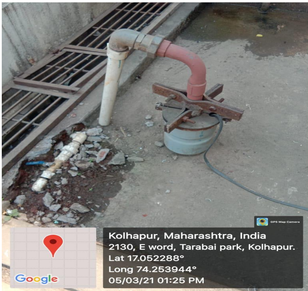
Picture 1. Borewell near the main building
