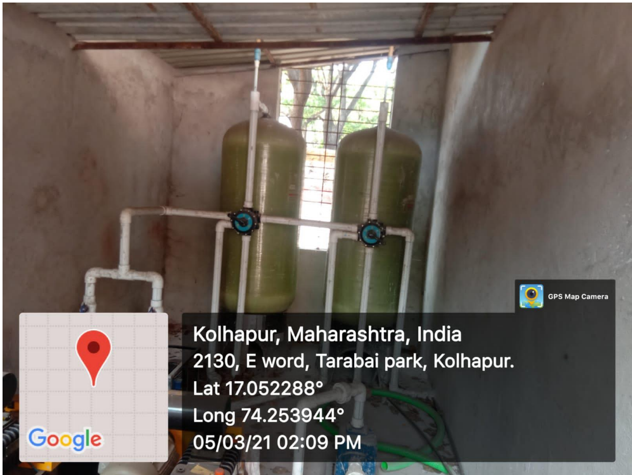
Picture 7. Waste Water Recycling Plant at the Ladies Hostel
