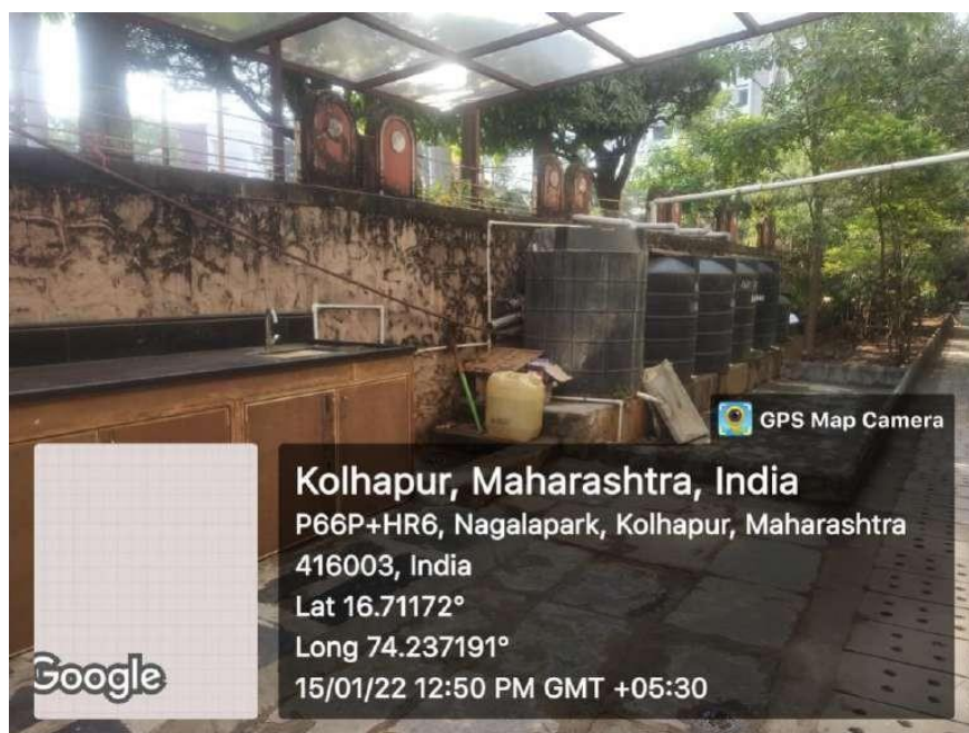
Syntax Water Tanks on the ground floor (Main Building)
