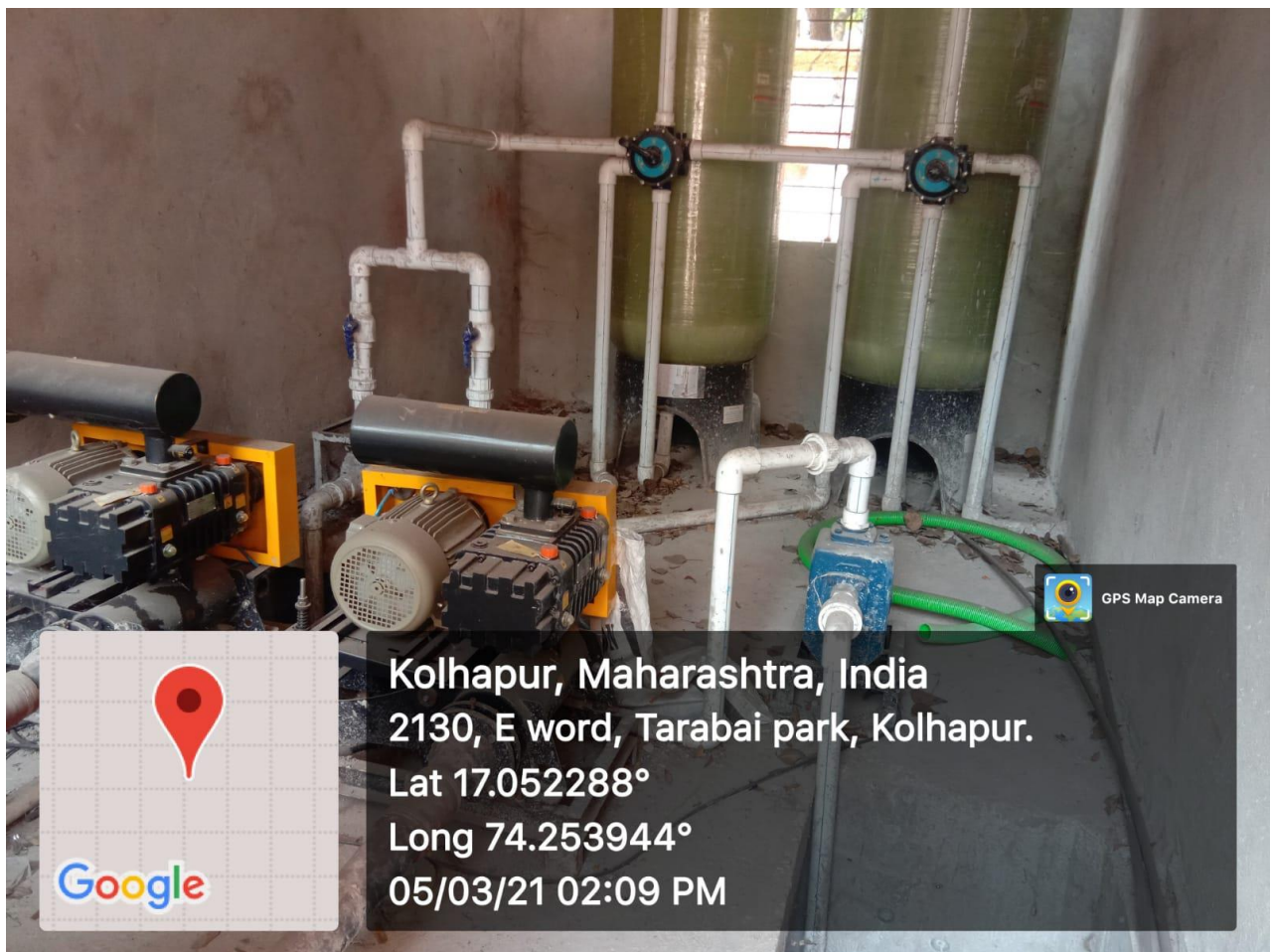
Picture 8. Waste Water Recycling Plant at the Ladies Hostel
