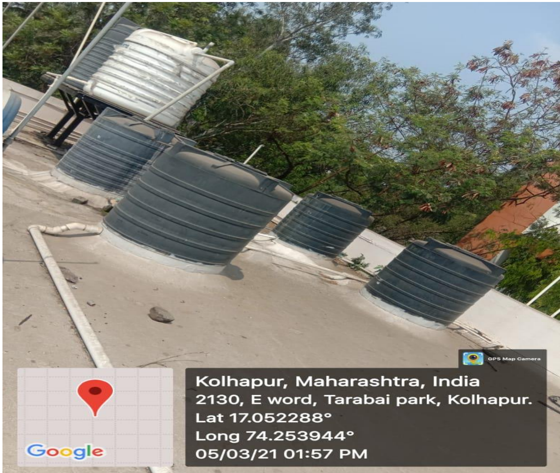
Picture 1. Water Tanks on the ladies Hostel 1
