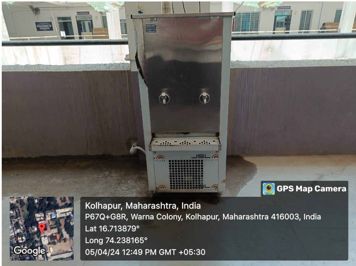
Picture 8. Drinking water facility at Physics department
