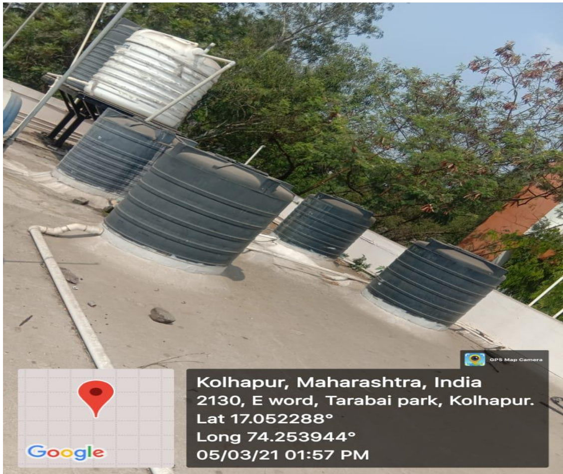
Picture 1. Water Tanks on the ladies Hostel 1
