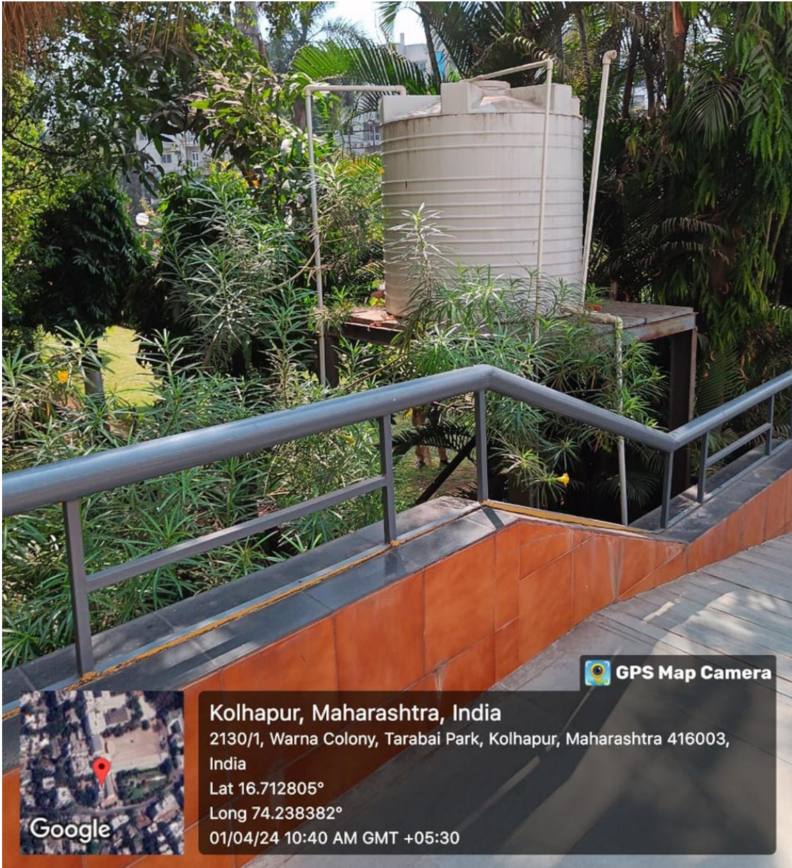
Picture 5. Tanks for water distribution in garden
