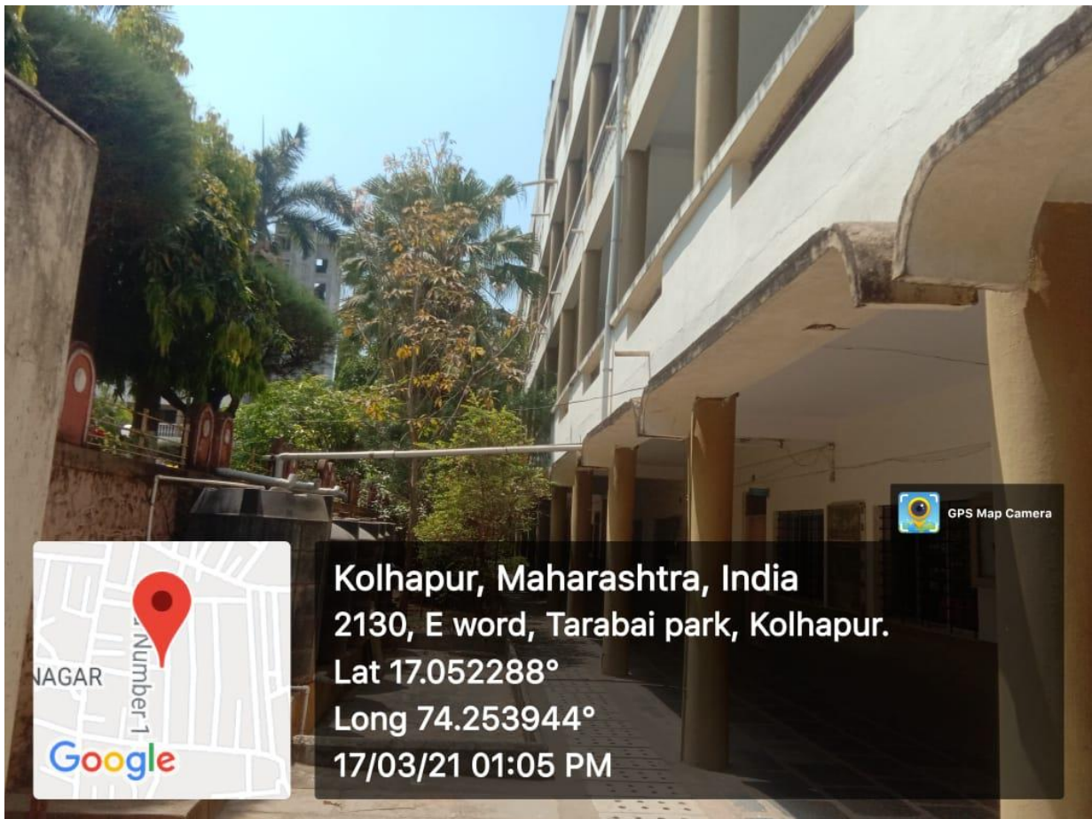
Picture 2. Rain Water harvested from the terrace and Channelized to the tanks
