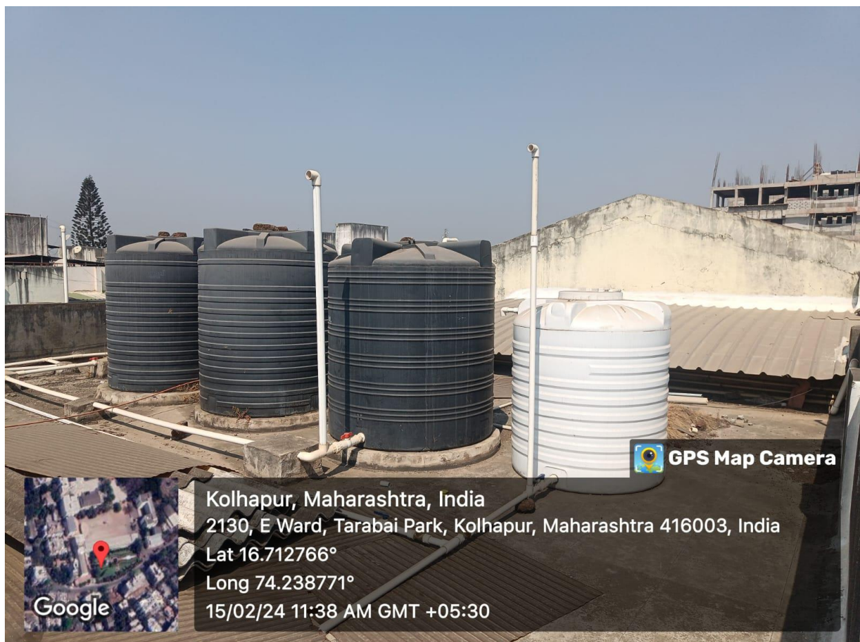
Picture 4. Water tanks for collection and distribution
