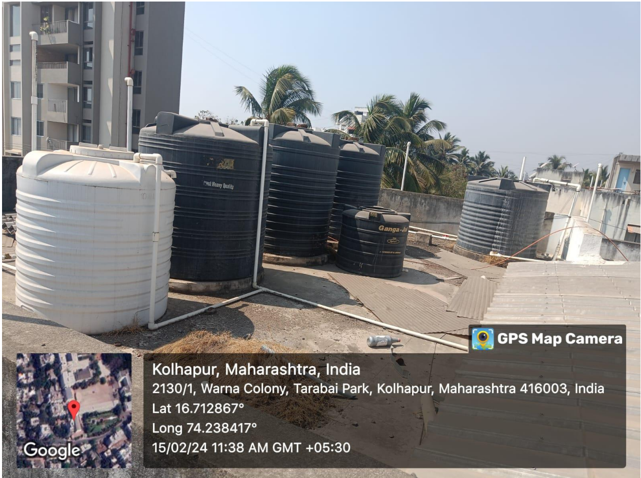
Picture 3. Water tanks for collection and distribution
