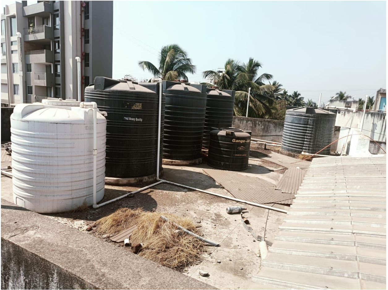
Picture 3. Water Tanks on the senior building
