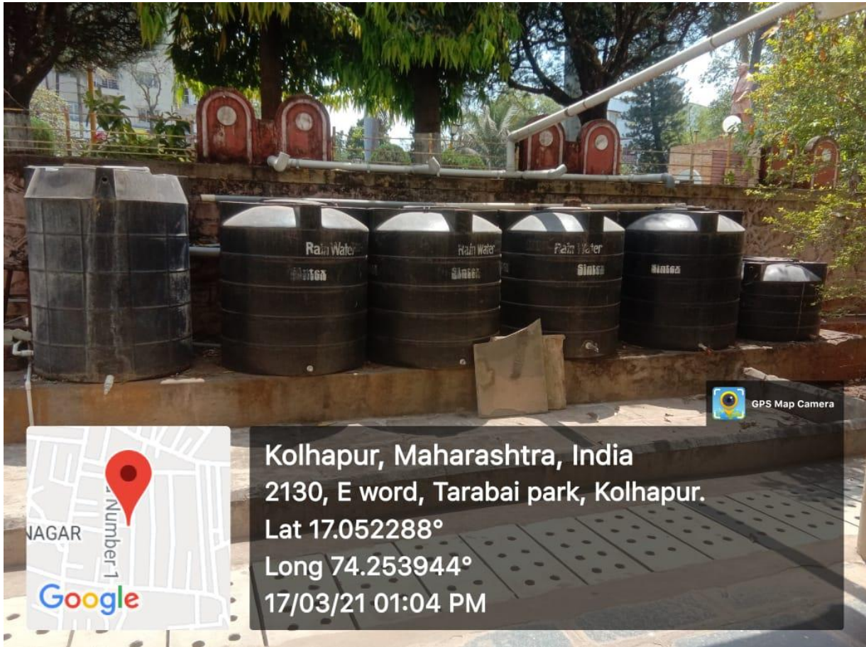
Picture 1. Rain Water stored in Water Tanks near Chemistry Lab
