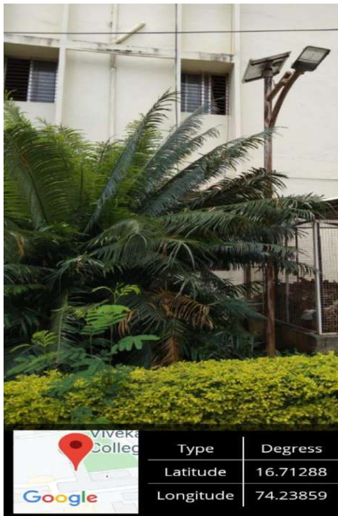
Plate No. 18: Solar Photovoltaic street lamps at Vivekanand College, Kolhapur
