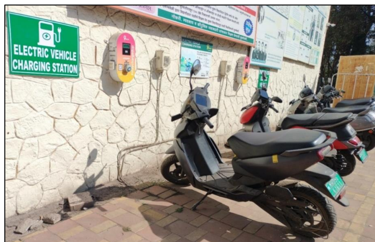
Electrical vehicles charging Station
