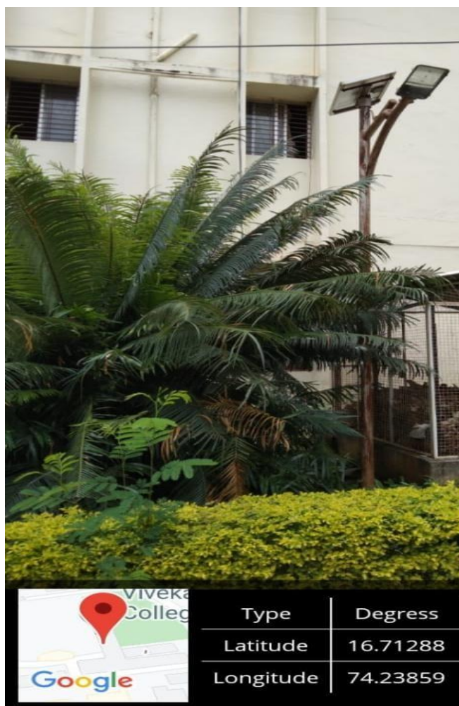
Plate No. 18: Solar Photovoltaic street lamps at Vivekanand College, Kolhapur
