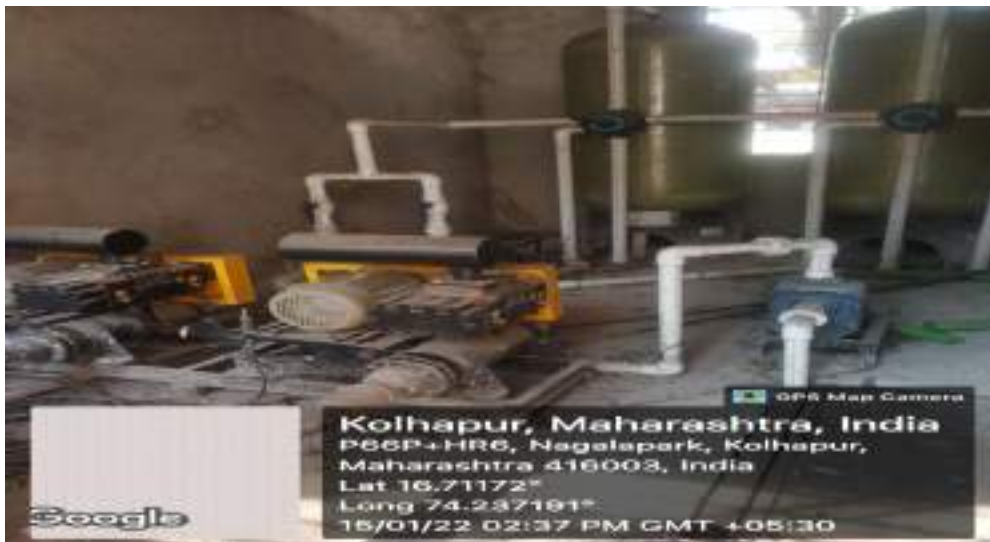
Plate No. 12 Waste water recycling unit
