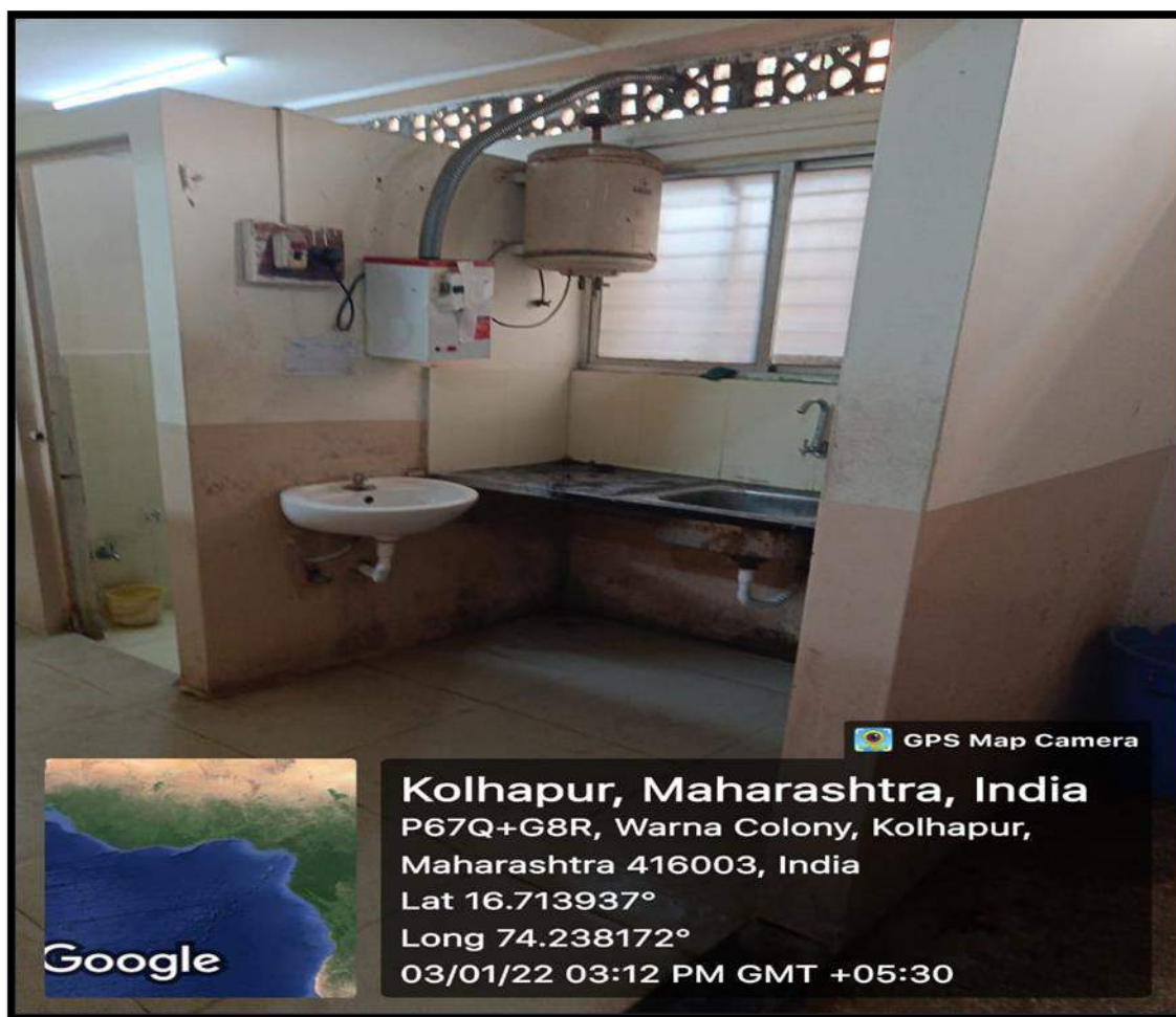
Plate No.9 Ladies Hostel Sanitary napkin disposal
