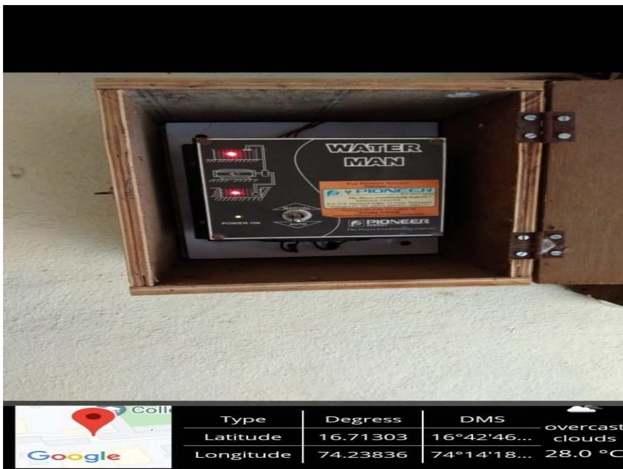
Plate No. 20: Sensor based Auto switch is used for bore well motor
