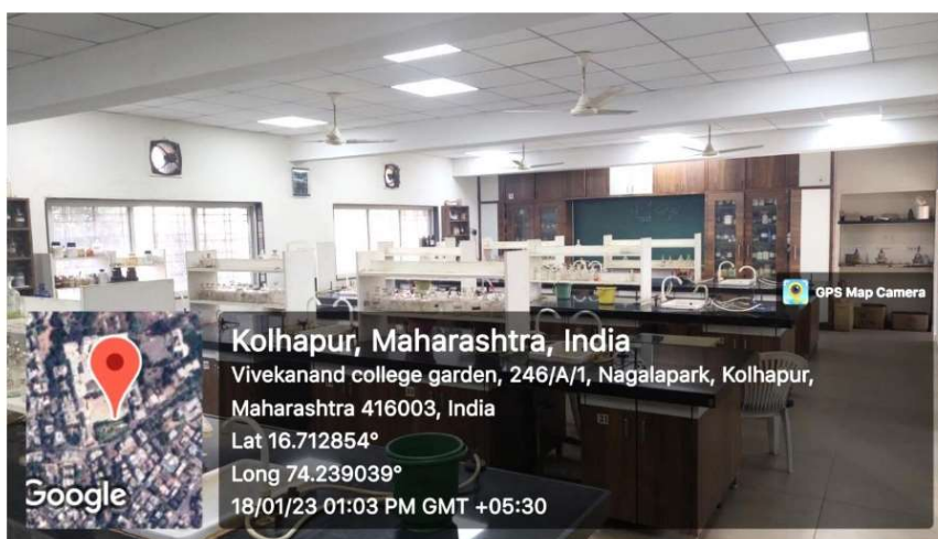
B. Renovation of Chemistry Laboratory: Renovation of Lab (9): Practical tables with storage cabinets, chemical storage cabinets, Green board, Flooring, Armstrong ceiling out grid ceiling, Decorative lighting and Aluminium ventilator etc.
